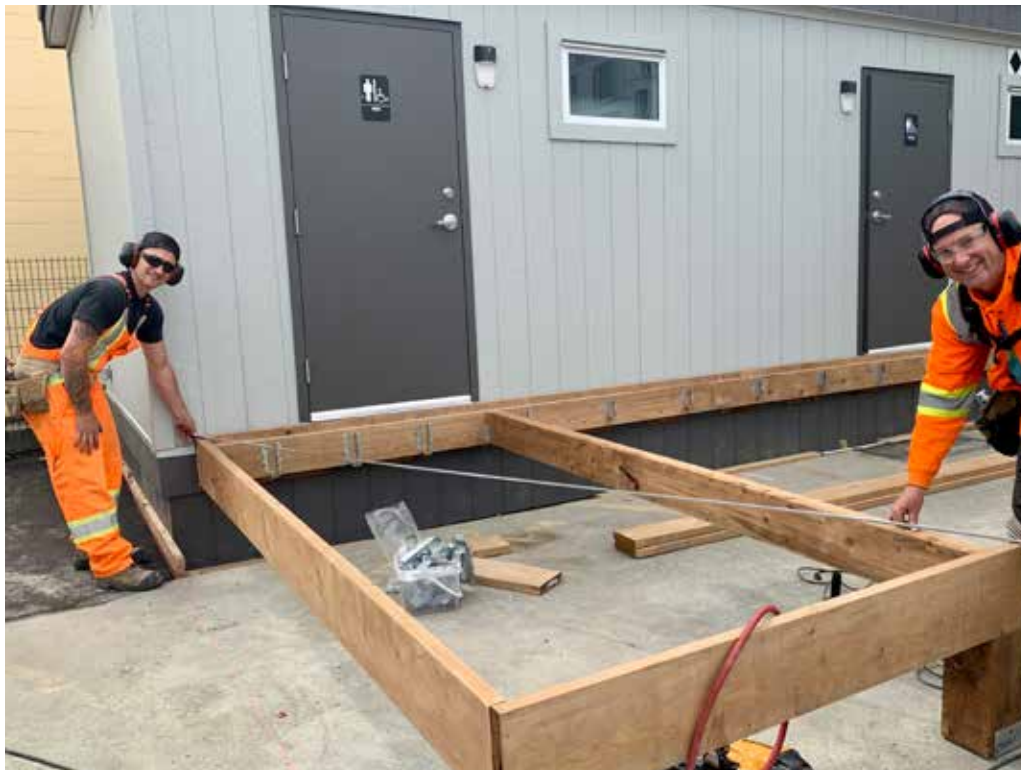
The Town replaced the public washrooms on Fourth Street near Beacon Avenue and built a new accessible ramp.
