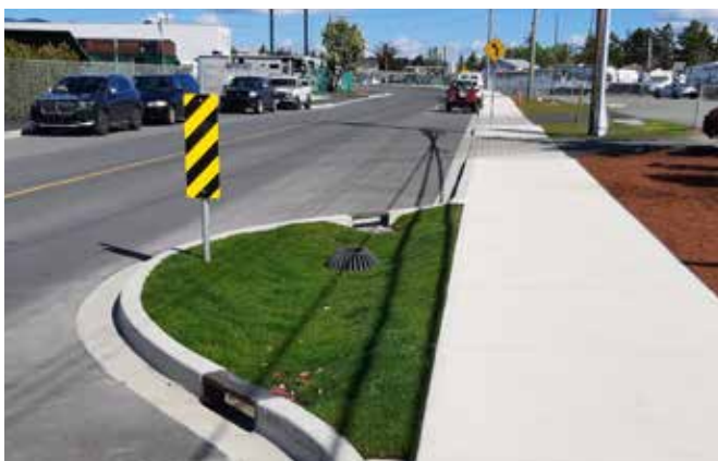
In 2023, the Town of Sidney made significant improvements to Galaran Road, including drainage and water works, new sidewalks, and road repaving.
